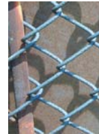
Before – exposed & corroded surface
